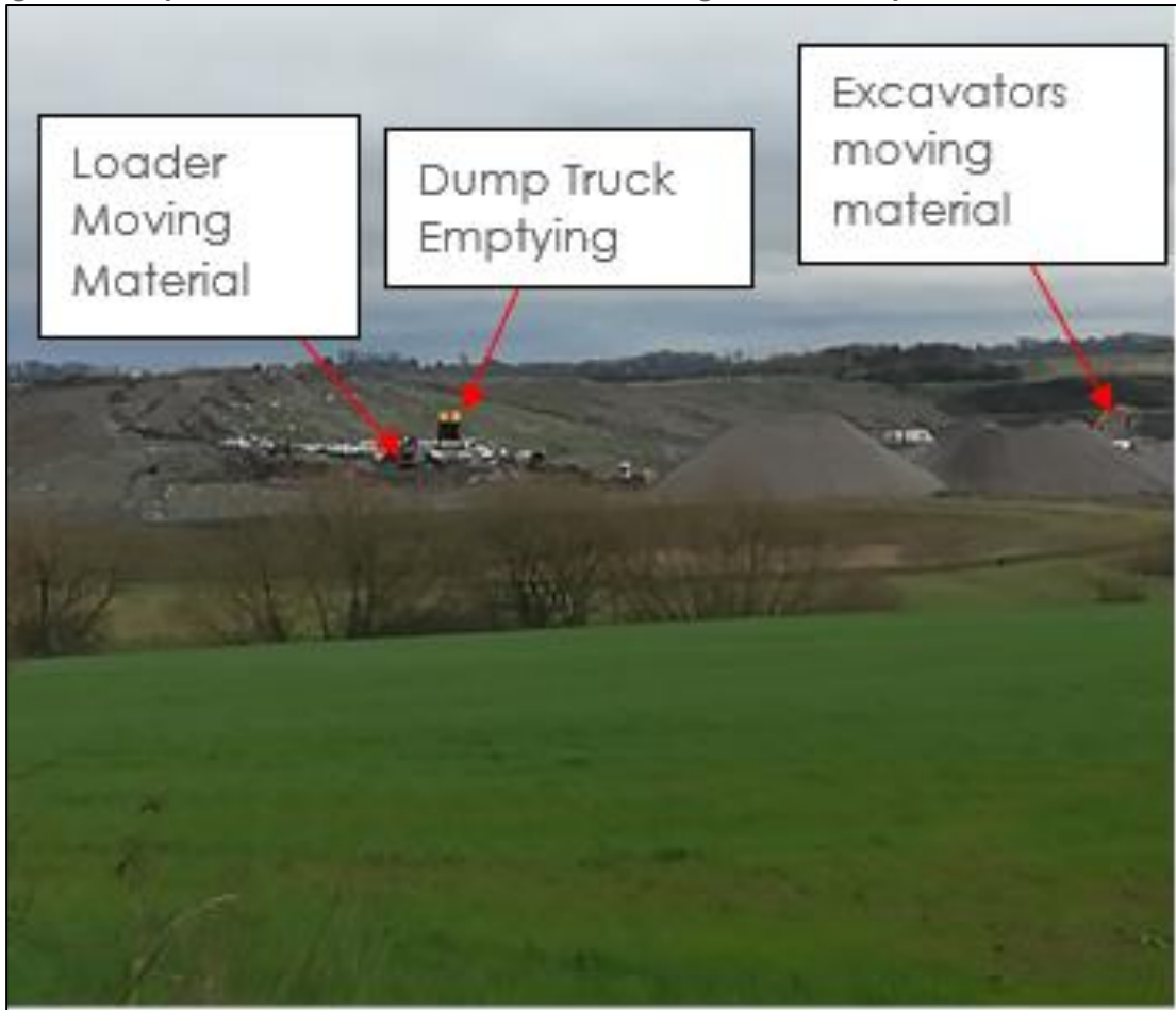
Figure 3-2: Operations at Hill and Moor Waste Management Facility
